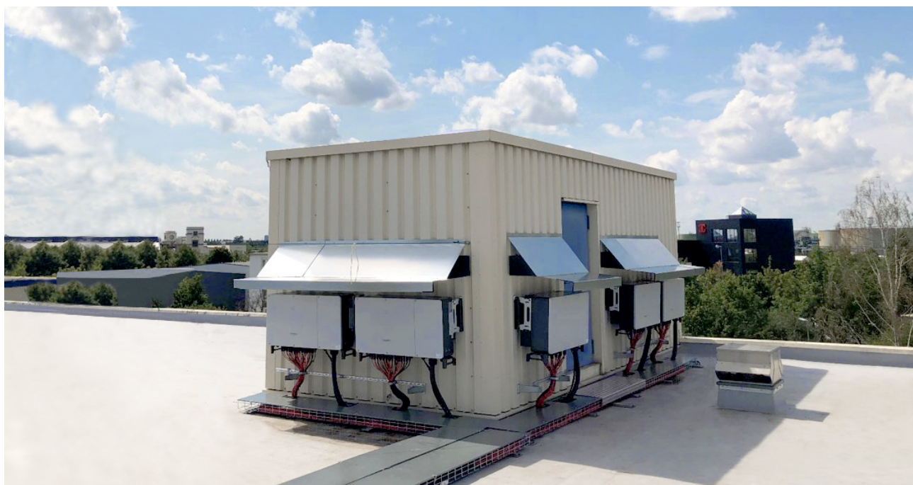
Fig.6 AC 500kW Rooftop PV Plant in Germany
